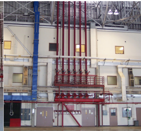
Red pipes of N211's new fire suppression system rise at the hangar's back wall to branch out to several key locations throughout the hangar.
